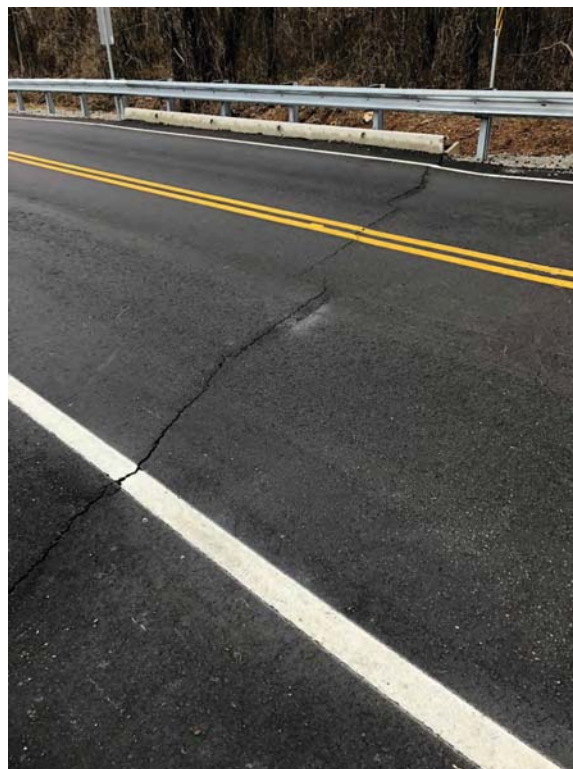
Pavement Cracking at East Abutment Connection
